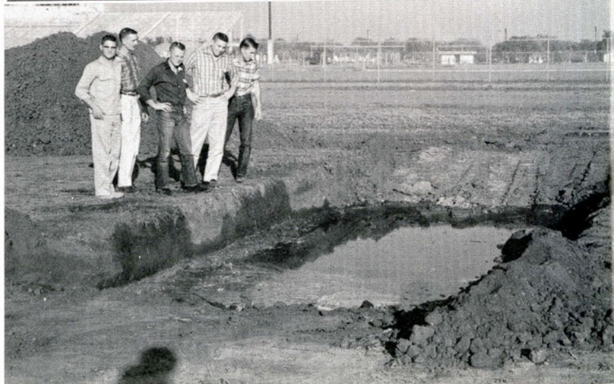
Many a good man and girl were lost at sea in the pit. The construction crew is shown looking over their work.
