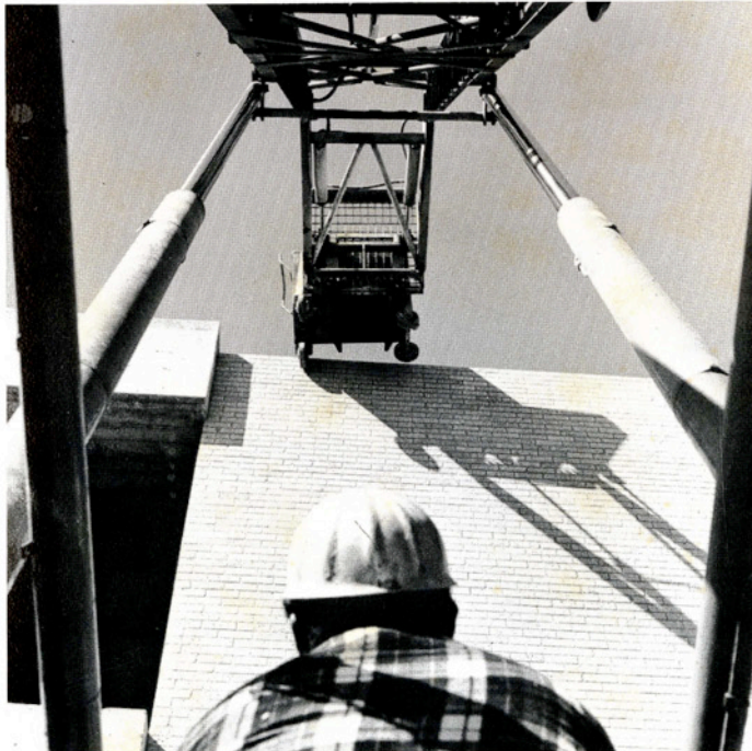
The new Earth Sciences Building is expected to be complete by the first summer session.
