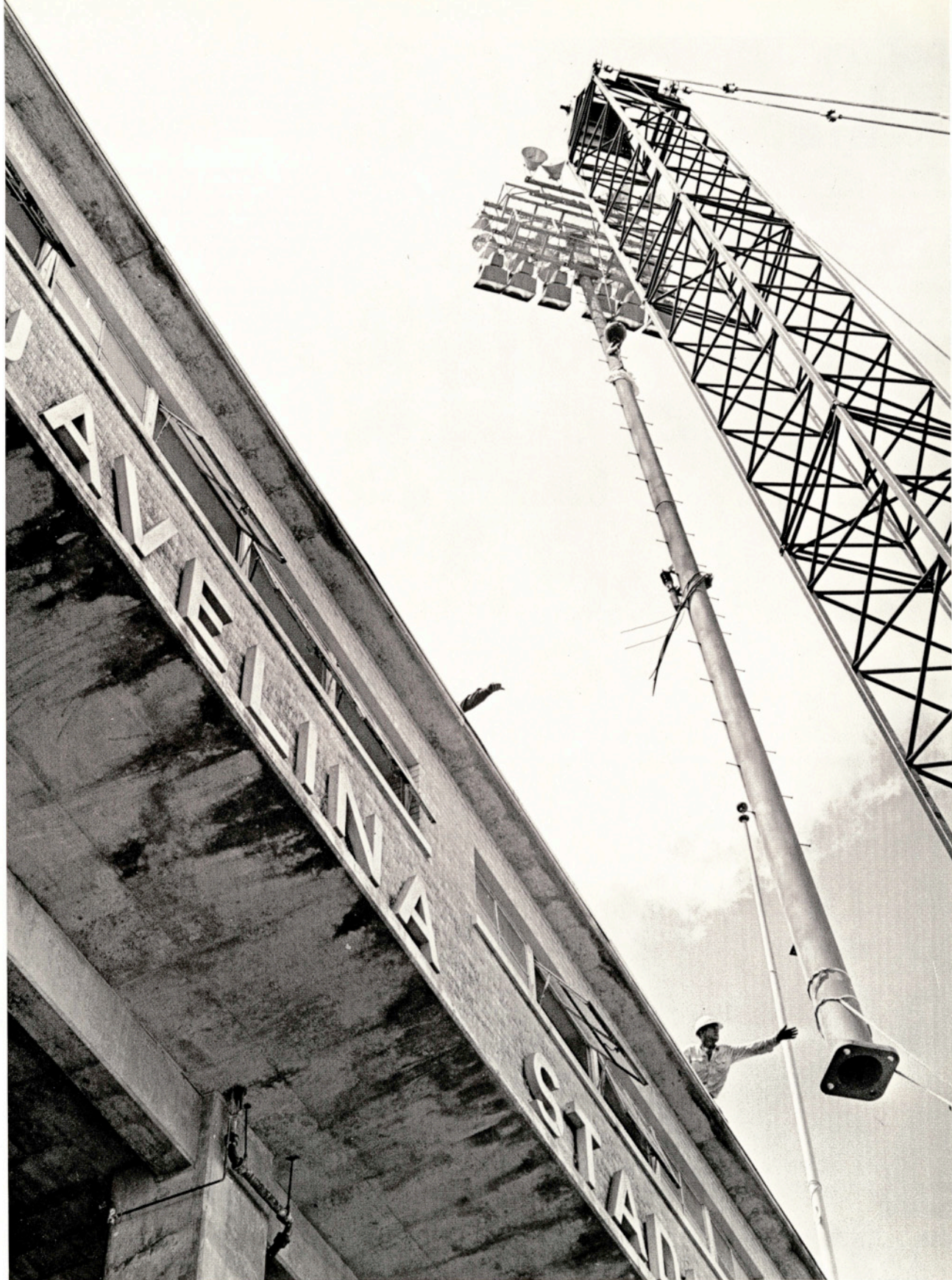
Stadium lights were swung into place during the summer as workmen replaced those destroyed by Hurricane Beulah in September, 1967.
