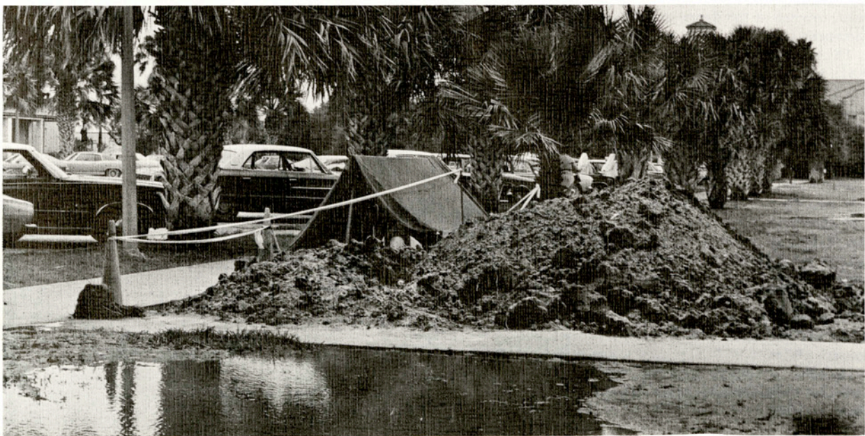
At the beginning of the fall semester, the University was switched over to a Centrex telephone system. The workmen installed an underground cable.
